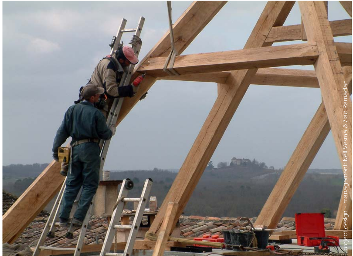
Seeing top quality craftsmanship, such as this oak-framed roof being built by local carpenters the Feltre brothers, is one of the best parts of Neil's work
